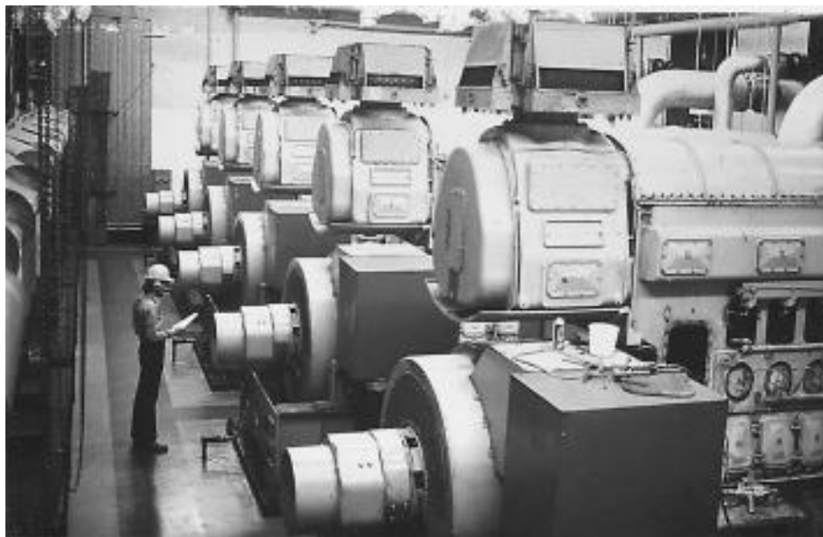
FIGURE 26-1 Ten-cylinder, dual-fuel-driven synchronous generator sets.
