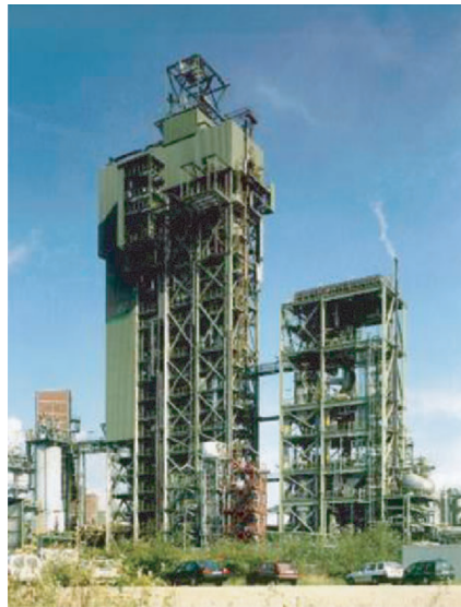
Fig. 8.1. HTW plant in Berrenrath, Germany
