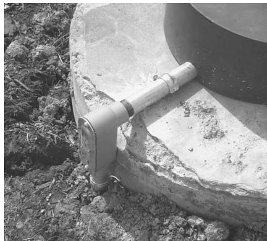
FIGURE 1-7 Exposed conduit is an easy target.
