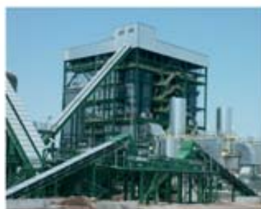
Strongoli, Italy, 2 x 24 MWe
