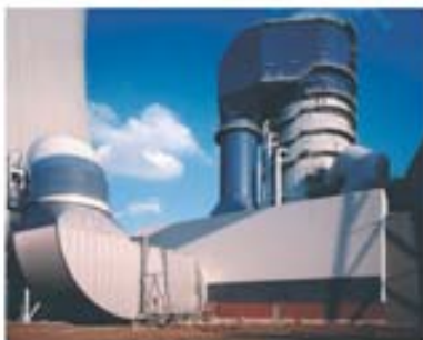
Rostock, Germany, 510 MWe 1.769.000 m 3 /h, Wet FGD
