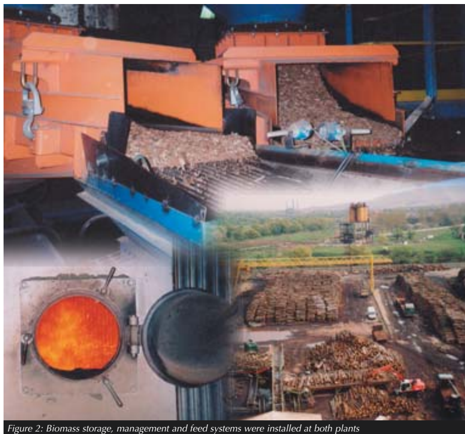
Figure 2: Biomass storage, management and feed systems were installed at both plants
